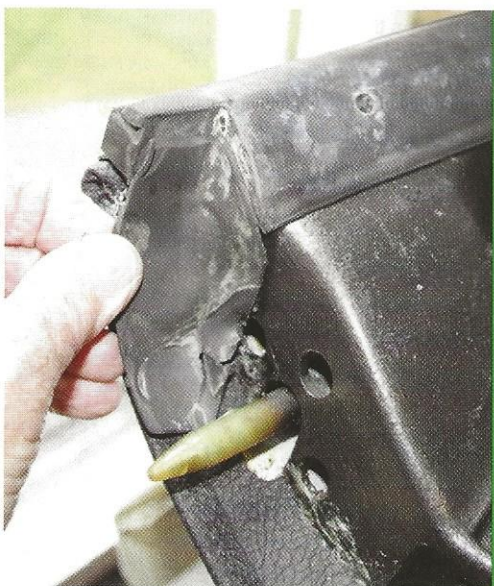
The window seals and gutters are fixed to the frame and the seal ends (tatty, new ones unobtainable) are glued in place and the end plates fitted
