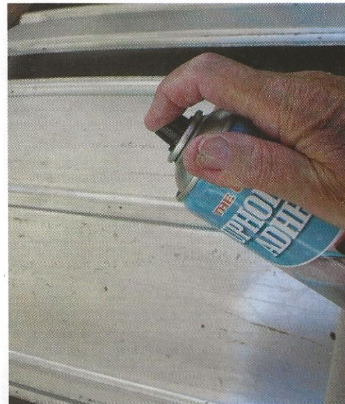
Spray glue is applied to both the aluminium panels and the linen before being stuck down, working from front to back and outwards to get a smooth finish
